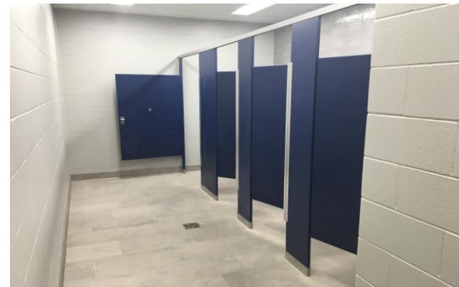
Toilet partitions are installed in all of the bathrooms throughout the school.
