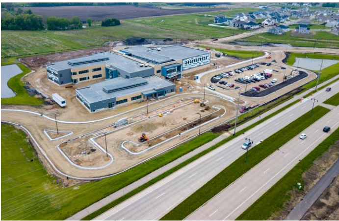
This aerial photograph from our drone last week shows that the school is only a little over a month away from completion! The asphalt will be poured next week to finish the parking lots.
