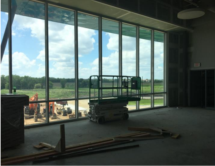
On the 2 nd floor, the loading dock has been replaced with the large windows. This will allow lots of natural light into the library!
