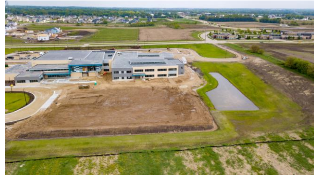
The lot for the basketball courts and playground is graded and ready to be paved!
