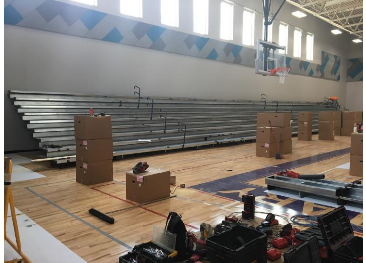
The bleachers in the gym are being installed, and the scoreboard will arrive next!
