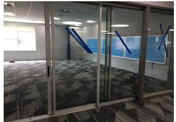
The glass sliding doors that separate classrooms from the hallway have arrived and are now being installed.
