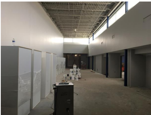
The ELRC is painted and ready to receive casework and ceiling grid!
