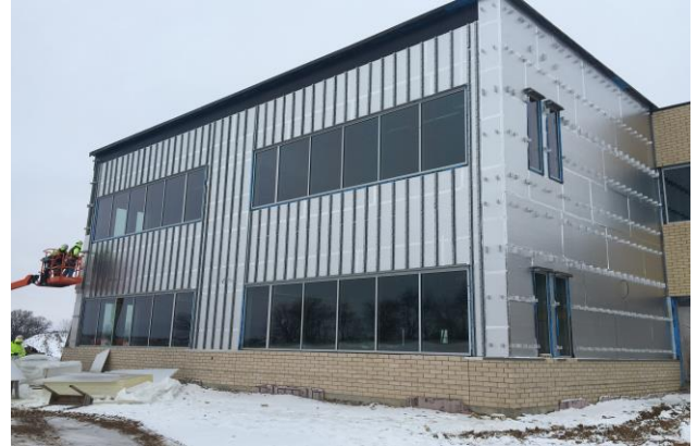
Metal panel clips and insulation are being installed around the classroom wings of the school, metal panels to follow next!
