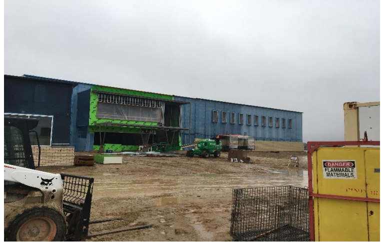
The main entrance of the building has been coated with the air vapor barrier, and the masons have installed low level brick around the gym!
