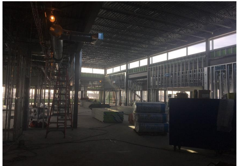
With the kindergarten/1 st grade wing drywall complete, crews will now start moving over to the 4 th /5 th grade area to start hanging drywall!
