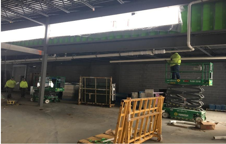
Plumbing is now being installed on the second floor above the cafeteria, with more HVAC ductwork and electrical wiring to follow.
