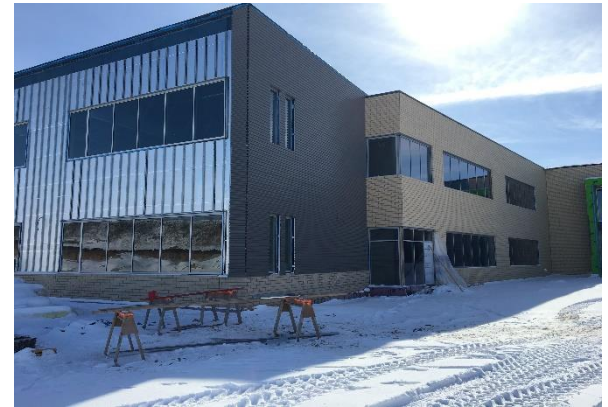
The metal panels are going up nicely, adding a sleek look to the building!
