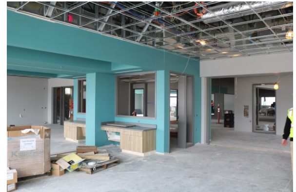
Painting is finished in the 2 nd /3 rd grade wing! Now ceiling grid is being hung and casework is being installed.
