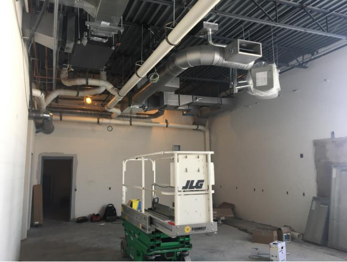
In the back of the kitchen, HVAC and plumbing is being rapidly installed to get ready for ceiling installation!
