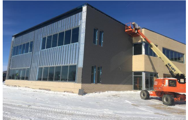
Now that the metal panel clips and insulation are in place, the metal panels are being installed around the classroom wings!
