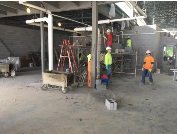
The masons are busy building the block walls for the 2 nd floor restrooms, kiln room, and art room!
