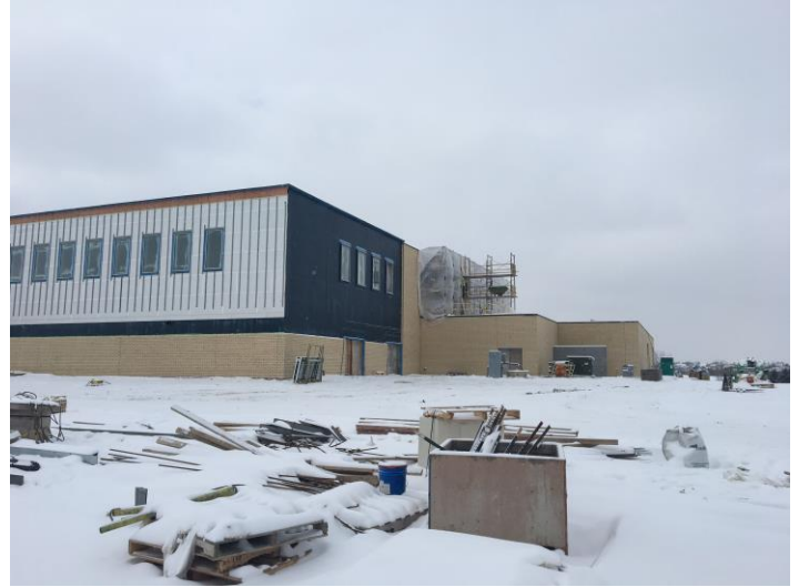
On the north side of the gym, masons are applying exterior brick. The silver "paneling" seen in this photo was installed last week, and it is the insulation for the metal panels.
