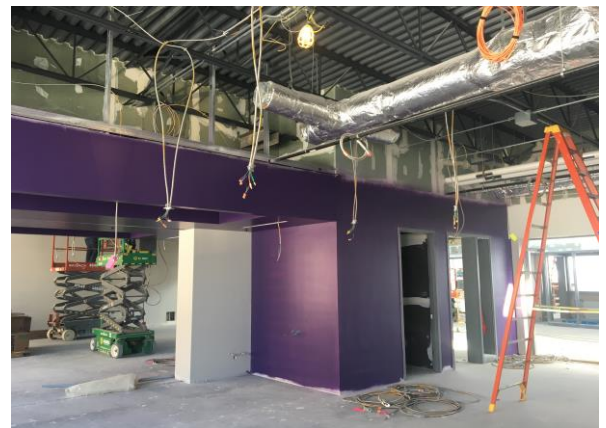
While this Kindergarten room is being painted, the electricians are busy pulling wire into the rooms!
