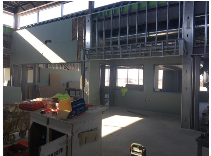
The crew has installed drywall in the classrooms of the 4 th /5 th grade wing, and they should finish up the wing next week!
