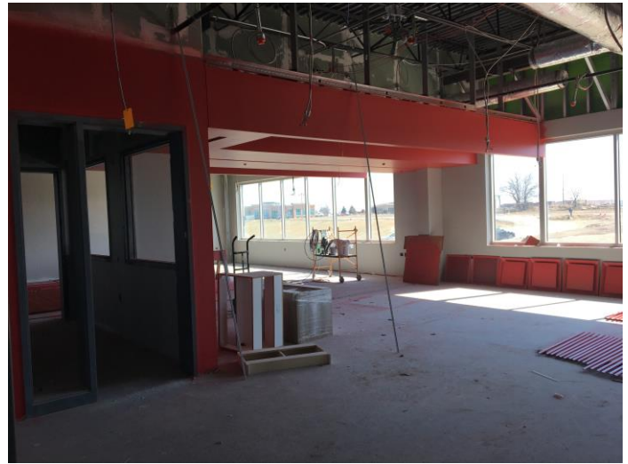
The 4 th /5 th grade wing is taped and the classrooms are now being painted! The hallway will be painted next week, and casework installation will begin after the wing is fully painted.
