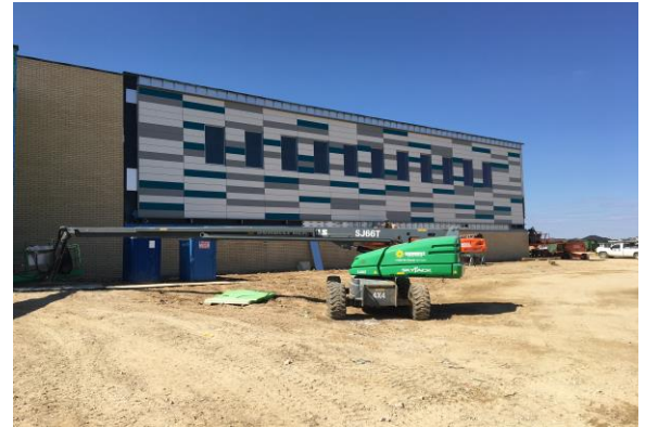
On the exterior of the gym, the colored metal panels have been installed! There are only a few spots left before all of the metal paneling is complete!
