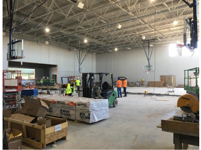
This week, the gym received basketball hoops, and more equipment will be installed in the weeks to come!
