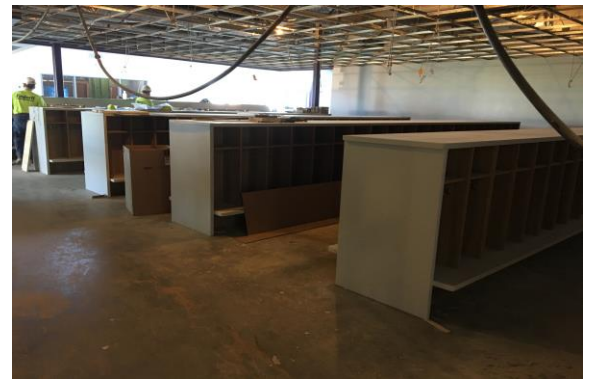
In the kindergarten/1 st grade wing, the carpenters have been busy installing cubbies!
