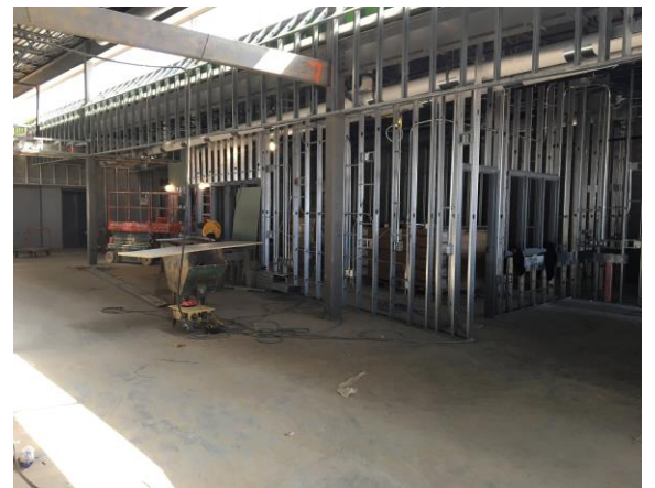
On the second floor, the walls of the art room, video room, and maker space have been studded and framed.
