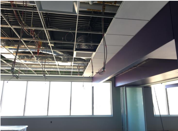
Ceiling tile has started to be dropped in the kindergarten/1 st grade wing. The tilers start on the edges and work their way towards the center of the room.
