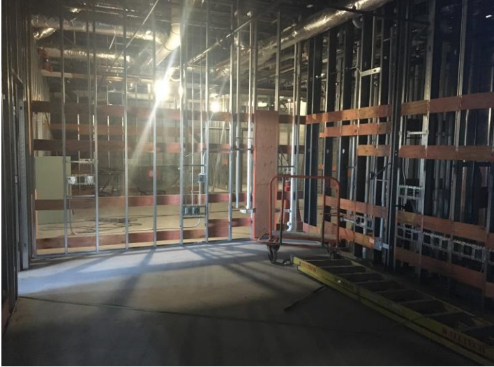
Here is a photo to demonstrate blocking! This is the nurse's office before the drywall goes up, and the blocking will be used to mount cabinets and drawers.
