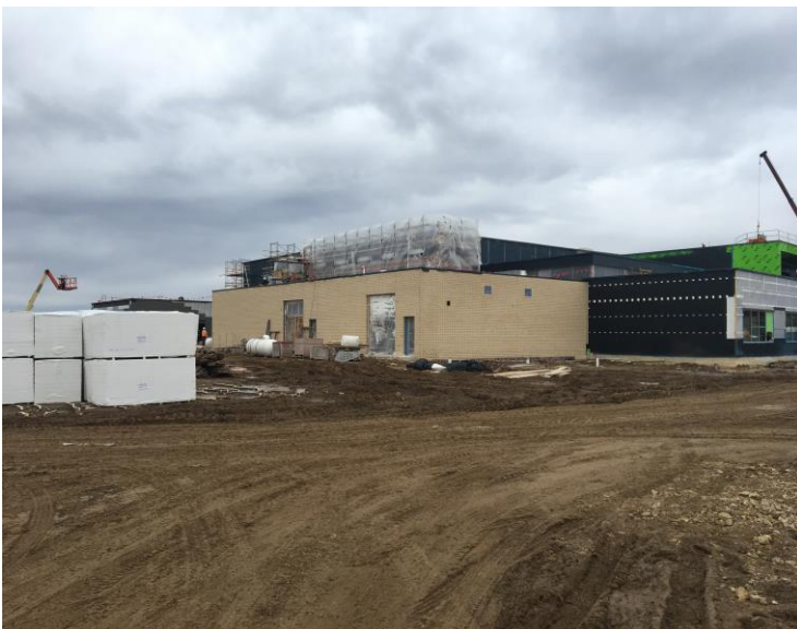
Masons are currently working on setting brick on the south side of the gymnasium.
