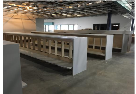
Last week, the casework arrived for the 2 nd /3 rd grade classrooms, so our carpenters have been installing the cubbies!
