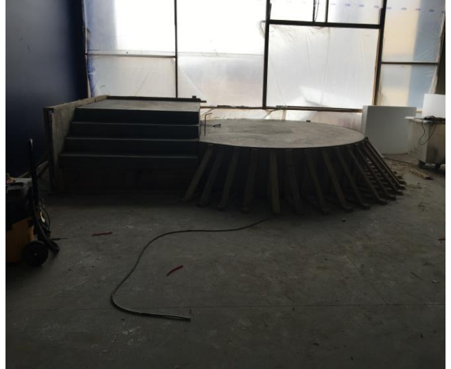
The concrete for the base of staircase 3 is poured, and the rest of the staircase will be installed next week!
