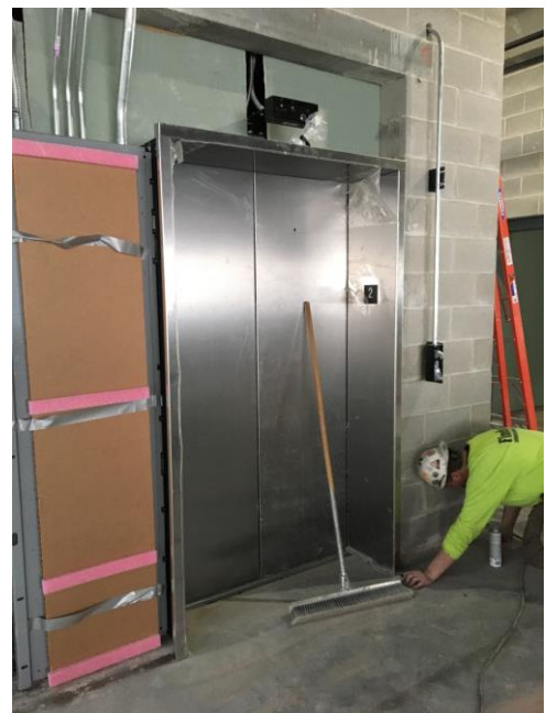
The elevator has been installed and the masons are laying block around the door frame.
