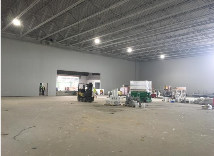
The gymnasium walls, ceiling and roof joist were painted. The HVAC overhead work will follow.
