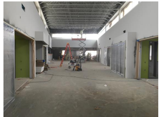
The kindergarten/1 st grade area is almost done being painted! After the painters are done here, they will move to the 4 th /5 th grade wing.
