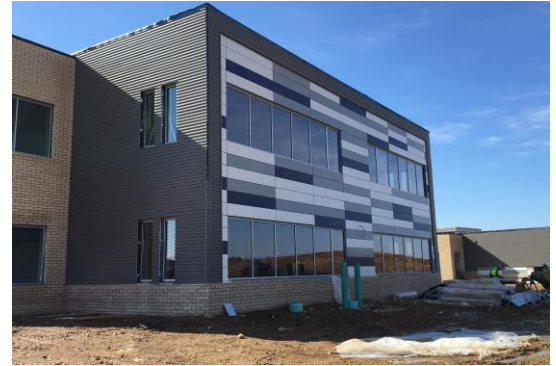
In the past couple of weeks, the composite metal panels have been installed. Here's a look at the colored panels outside the 2 nd /3 rd grade classrooms!
