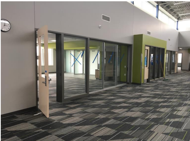
Carpet installation is finished in the kindergarten/1 st grade wing, and the wing is complete except for minor touch-ups! The sliding glass doors, the door hardware, and the clocks were all also put in this week!
