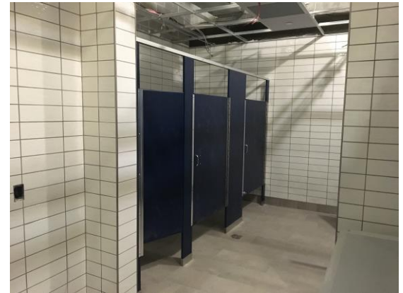
Toilet partitions have been installed in the cafeteria bathrooms, and will next be installed in the classroom wings.
