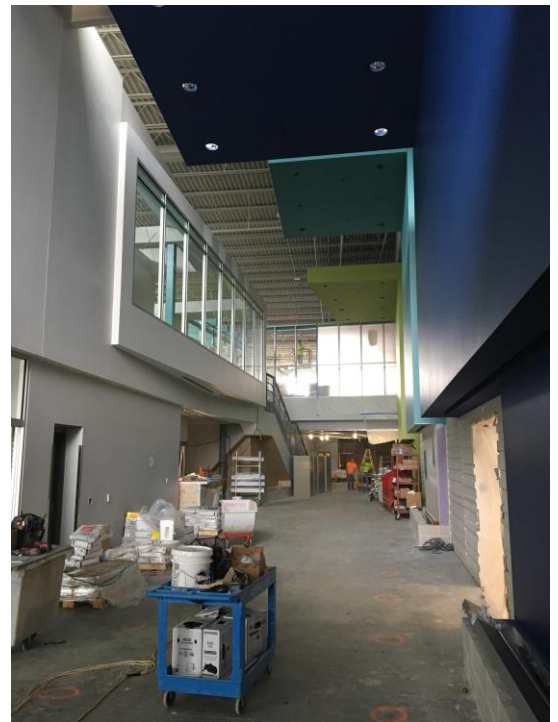
In the main entrance hallway, the cloud soffits are painted. They are painted the same colors as the classroom wings!
