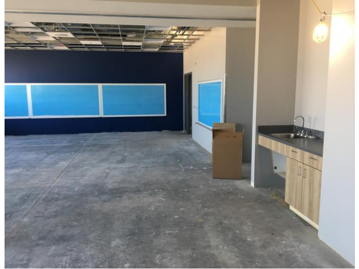
Whiteboards and casework have been received in the ELRC. Next, flooring will be installed along with ceiling tile!
