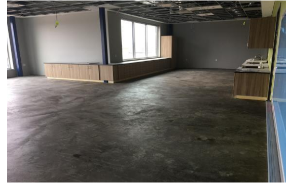
In the art room, the casework is installed and the concrete floor is being sealed.
